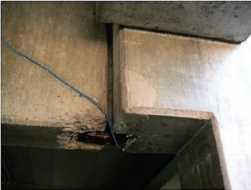
Figure 7.12 Spalling of cover concrete around a steel plate connector due to corrosion. The cover distance was 12 mm minimum. The age of the building was about 15 years when the photograph was taken.
