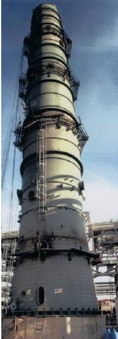
Vertical vessel tower
