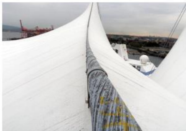
Figure 3. Ridge cables supporting the fabric.
