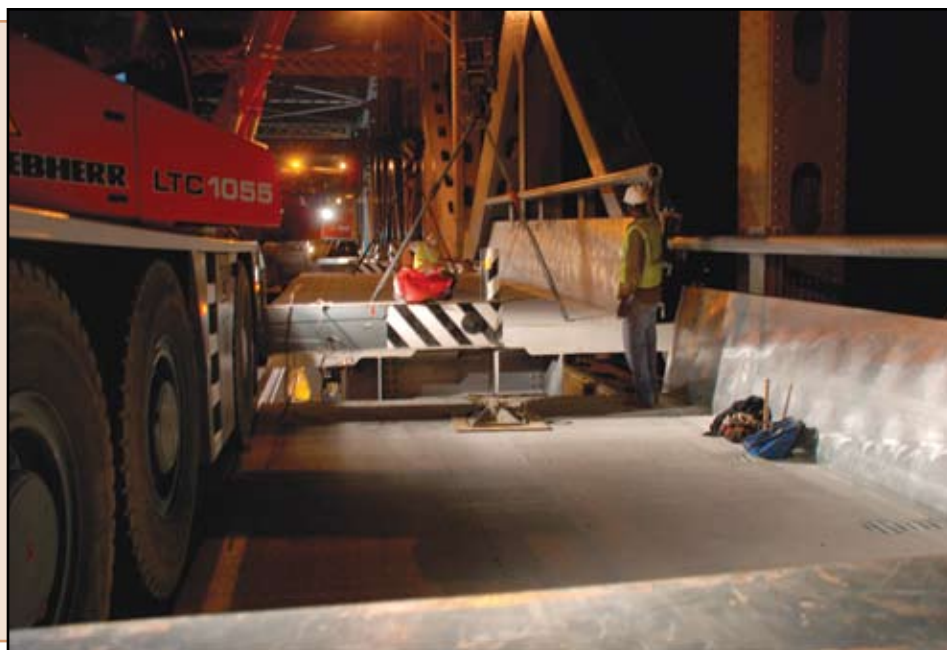
Installation of exterior precast deck panel, including permanent steel barrier, at main span, ready for vehicles to ride on in the morning.
