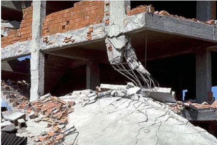
Details of damage to third-story column of Building B
