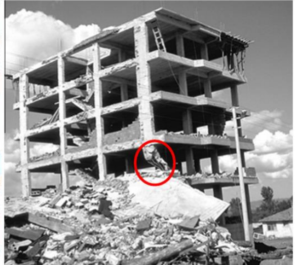
Column loss on third story of a building during 1999 Izmit Earthquake, Turkey |
