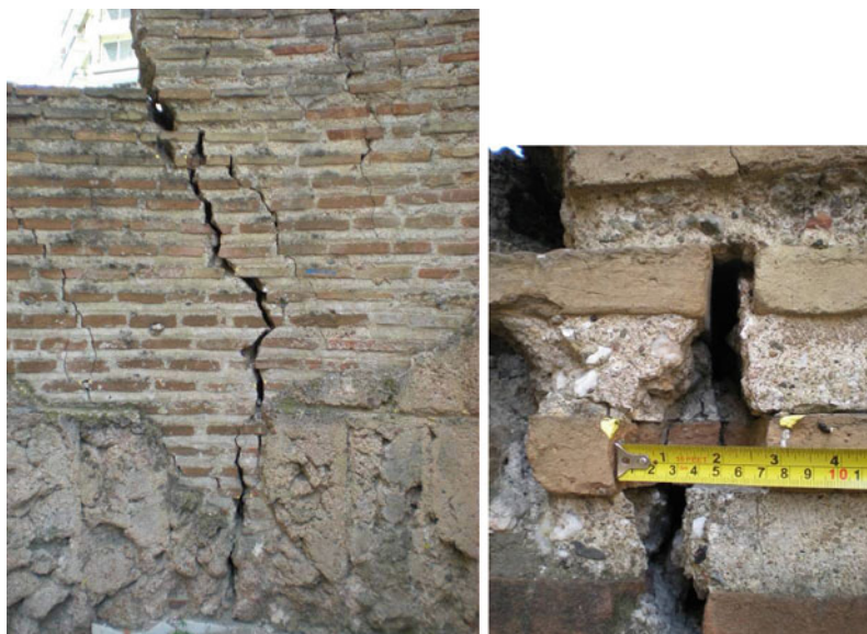
Fig. 2 Galerius palace ensemble, third century AD. Cracks filled with flowable lime-based mortar
