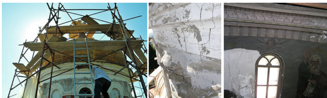
Fig. 6 The damages of the dome of the monastery at Andreas in Mount Athos before repair intervention (Photograph courtesy of G. Mitolidis)
