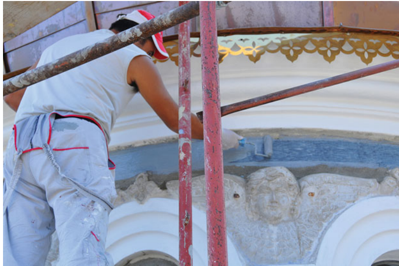
Fig. 7 The use of CFRP for strengthening the base of the dome of St Andreas in Mount Athos, 2011 (Photograph courtesy of G. Mitolidis)
