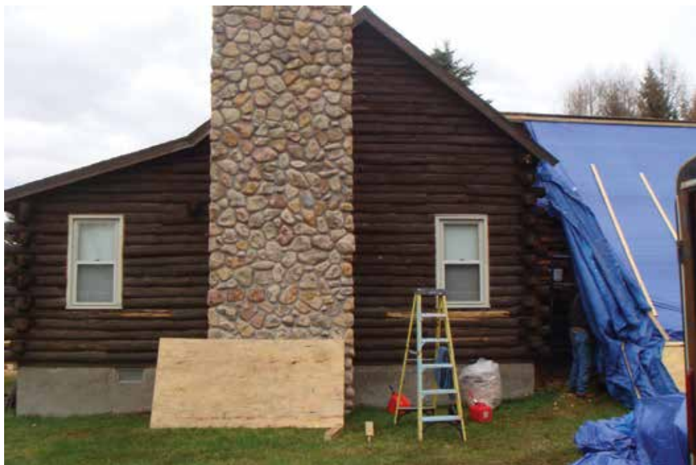
Figure 1. Elevation of deteriorated log wall.
