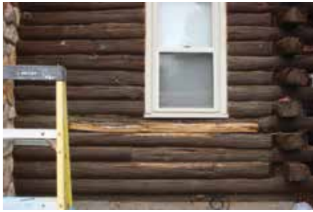
Figure 2. Close-up of rotten logs.
