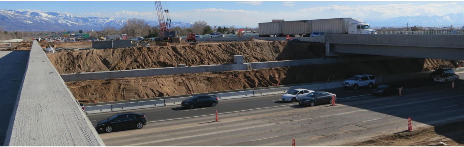
◀ The sliding system involved an end diaphragm with the stainless steel slide shoe on Teflon bearing pads.
