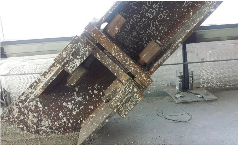
▲ A tension release at a braced end-plate connection.
