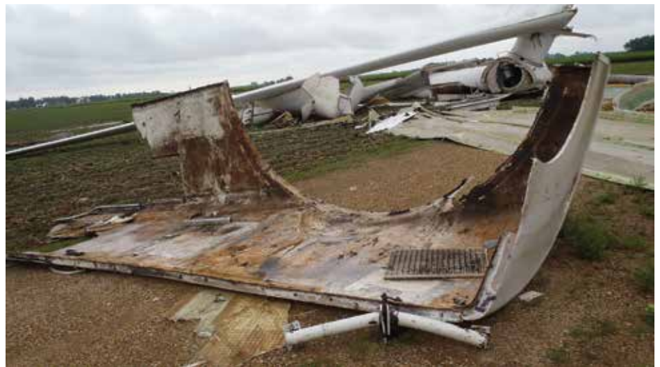
Figure 4. Localized debris field following wind turbine over-speed, due to mechanical failure within the nacelle. Remnants and evidence were found 650 feet (198 meters) from the tower base.
