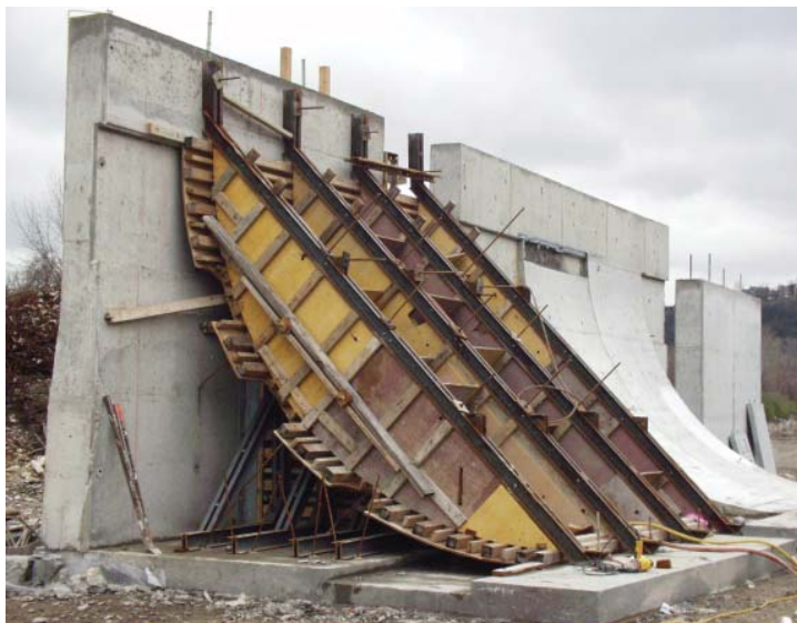
Figure 1: Curved form mock-up for the Urban Carpet Roll a featured curved concrete structure on the Rosenthal Center for Contemporary Arts. Concrete contractor Baker Concrete Construction, Inc.
