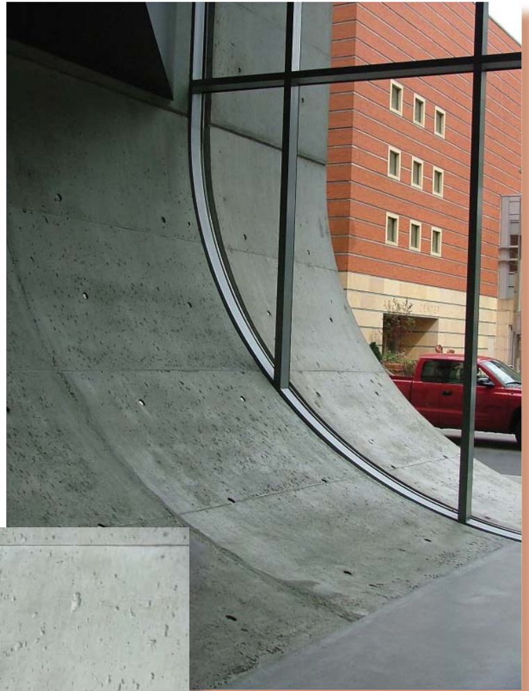
Figure 5: The Bungholes in the concrete caused by non-escaping air bubbles on the horizontal portion of the form where used to enhance the architectural concrete
