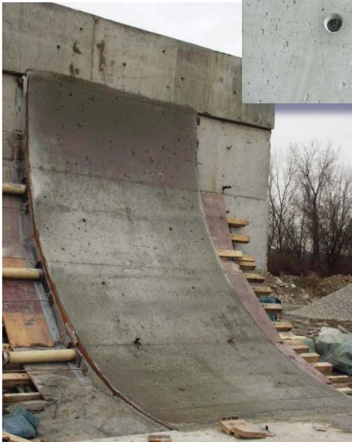
Figure 3: The mock-up process allowed for a successful installation process, the formwork, concrete mix and construction procedures were resolved. Concrete contractor Baker Concrete Construction, Inc.
