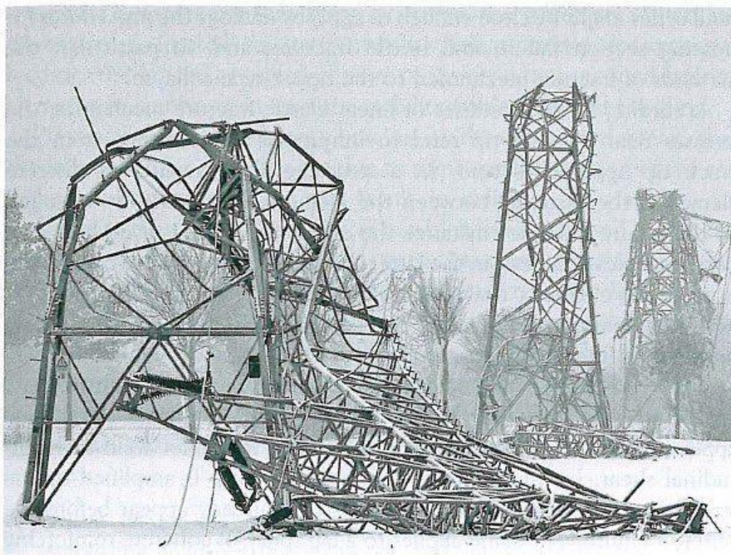
Fig. 2.3 Domino-type collapse of overhead transmission line towers triggered by ice accretion (Germany, 2005). (Source: picture-alliance/dpa/dpaweb. Photograph: Franz-Peter Tschauner, © dpa)
